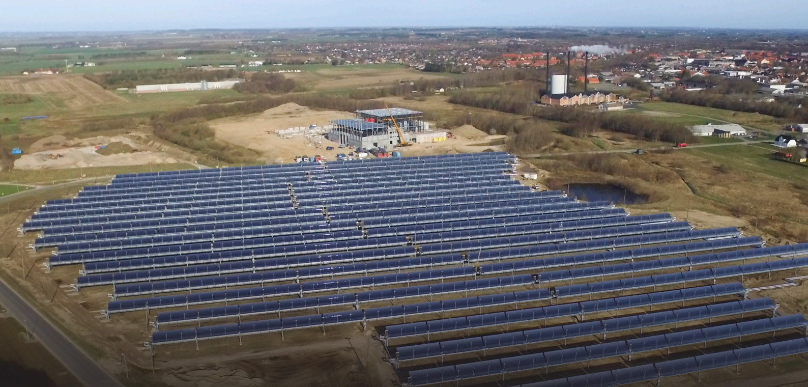
Brønderslev Forsyning, Varme, with 5000 DH customers, has one of the most energy-efficient CHP plants globally. It combines concentrated solar heating (CSP) with wood chips and converts the energy into electricity and DH via a so-called ORC system (Organic Ranking Cycle).
